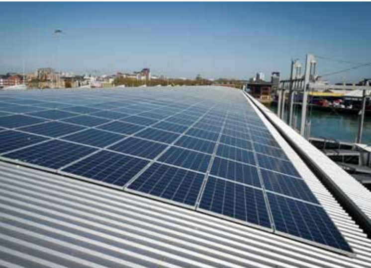
Solar arrays installed across the Port of Southampton
